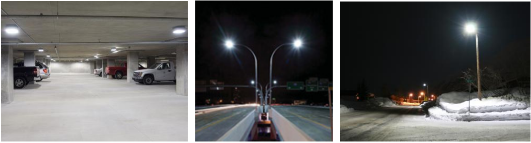
Figure 5. Installations of Indoor and Outdoor LEDs Lighting Demonstrations in the US
